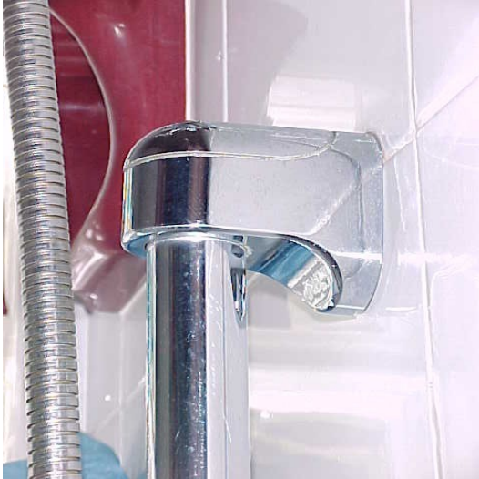
Bottom part of Shower Head (Free of corrosion)
