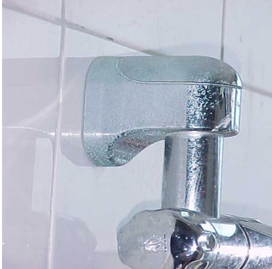
Corroded Shower Head Holder from Chlorine vapour
